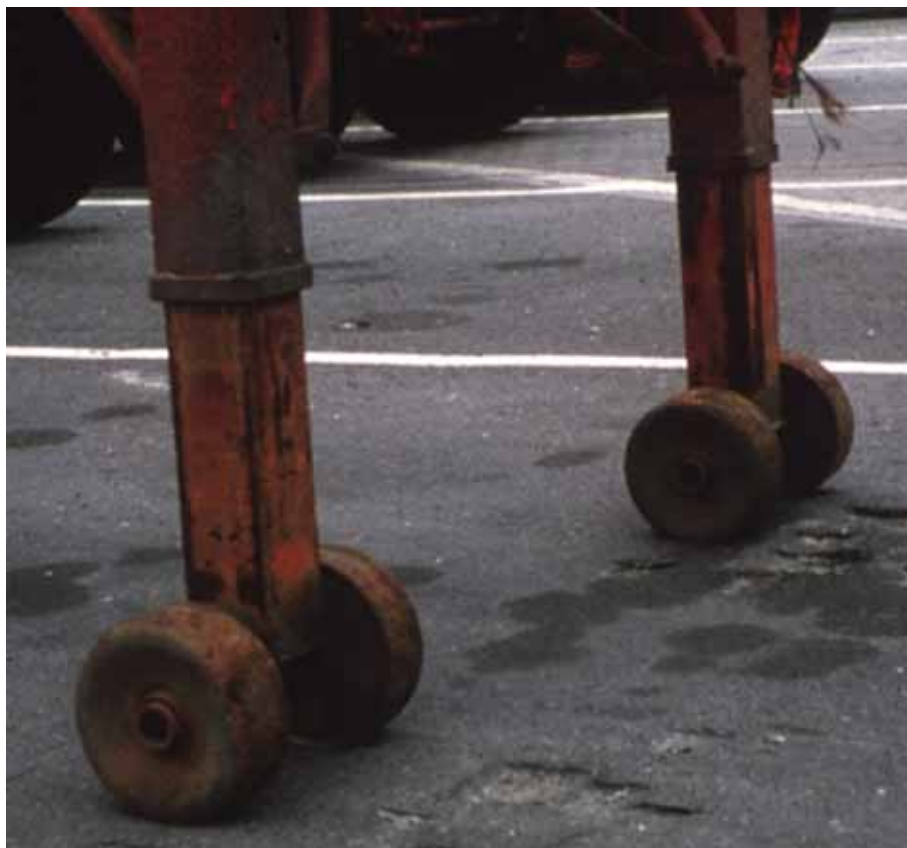
Figure 10. These trailer jockey wheels have indented the bituminous material surfacing.
