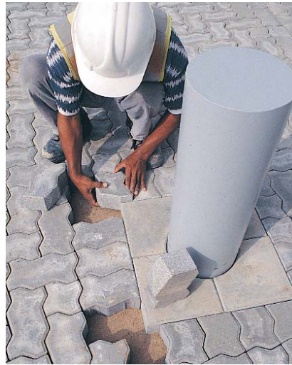
Figure 13. Cut pavers were fitted around concrete collars at bollards and at utility structures.
