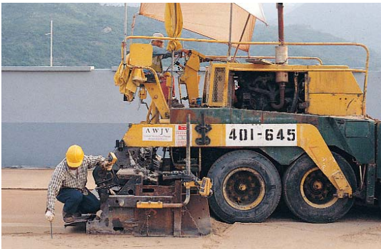
Figure 7. A sonic-controlled asphalt machine accurately placed, \frac{3}{4} in. (20 mm) thick bedding sand layer over a smooth CTB surface.
