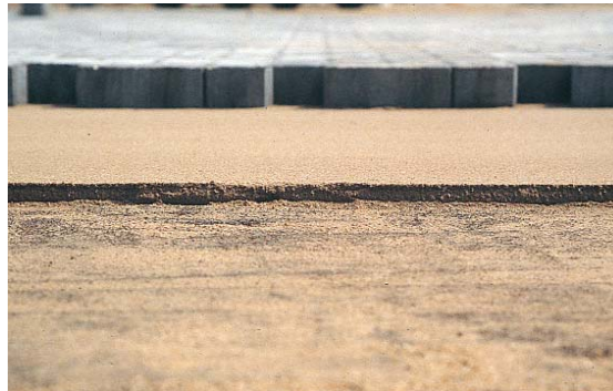
Figure 8. The screeded bedding sand maintained a consistent thickness since the surface of the CTB met tolerances for smoothness.
