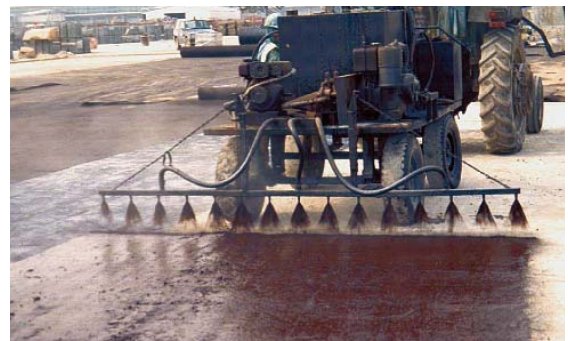
Figure 6. A bitumen tack coat secures geotextile in place over the CTB. A thin layer of sand was then spread to keep the bituminous material from sticking to boots and tires.
