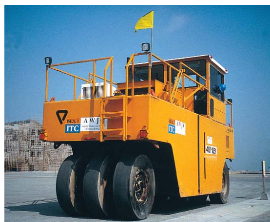
Figure 18. This 44-ton (40 T) machine rolled the completed surface of the pavers (prior to application of the sealer) to prove that they were seated and that the joints were full of sand.
