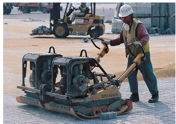
Figure 15. 9,000 lbf (40 kN) plate compactors were used to compact the pavers into the bedding sand, then again to compact the joint sand into the joints. Two were joined for greater efficiency.
