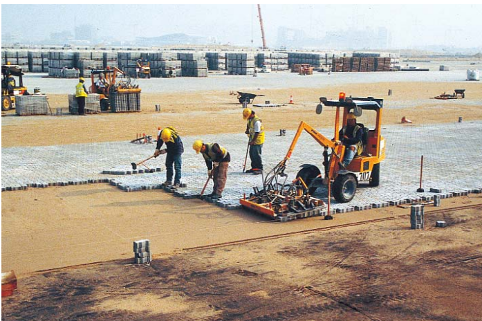
Figure 10. Mechanized installation accelerated paving by using three machines to place layers of pavers in their final herringbone laying pattern. Note the bundles of pavers in the background and the crew adjusting joint lines and tightening each layer against its neighbors.
