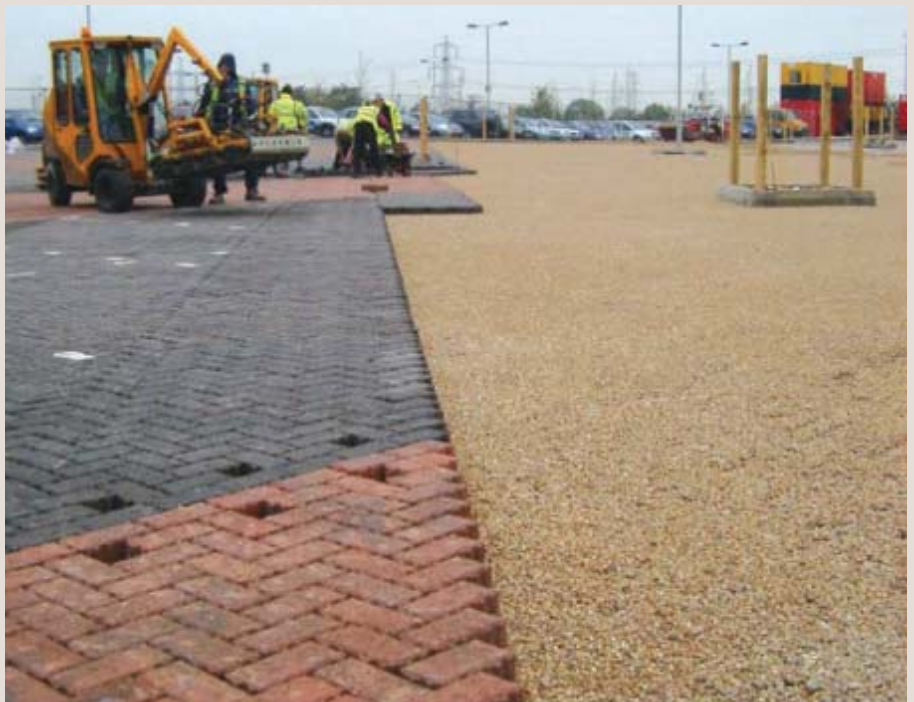
Figure 42: Machine laying of concrete paving units offers a particularly efficient solution for permeable as well as conventional block paving.
