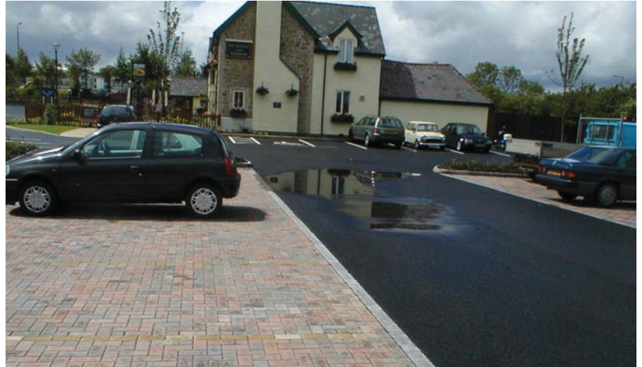
Figure 5: comparing impermeable paving (right) and concrete block permeable paving (left) under similar rain conditions.
