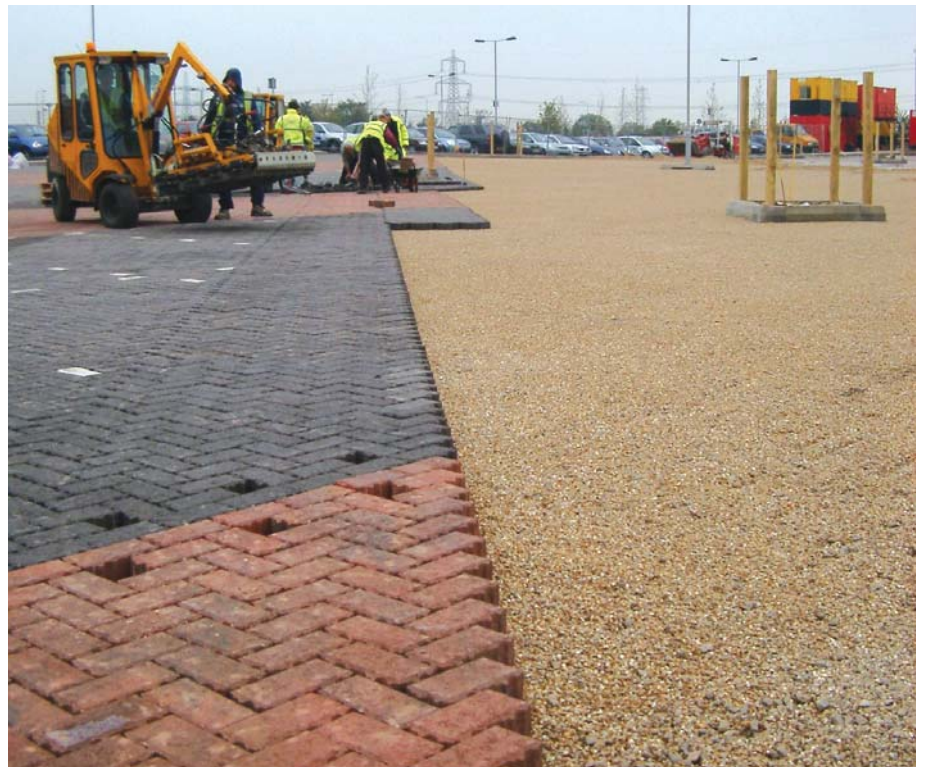
Figure 34: Machine laying of concrete paving blocks offers a particularly efficient solution for permeable as well as conventional block pavements.
