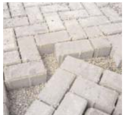
At Santos, rectangular paving blocks with oversized spacers were used as the surface to the permeable pavement.
