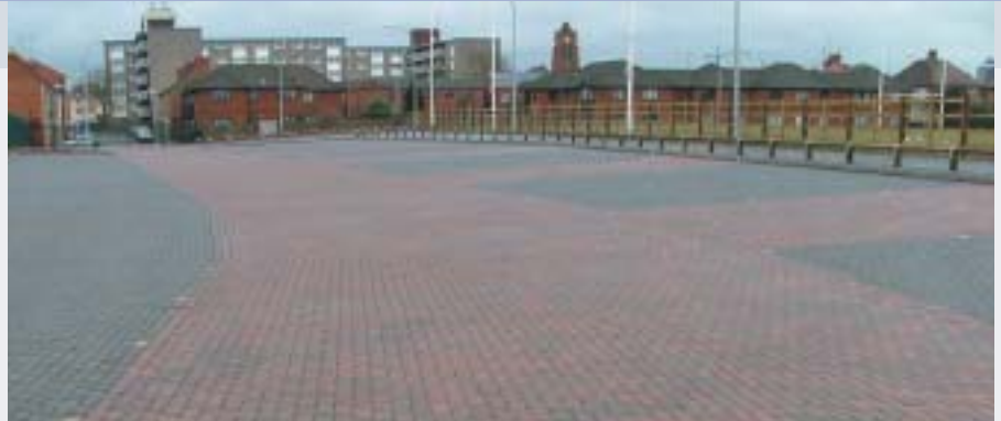
In Northampton, over 50,000 m 2 of CBPP attenuates and treats surface water before discharge to watercourses (photo courtesy of Mowlem plc).
